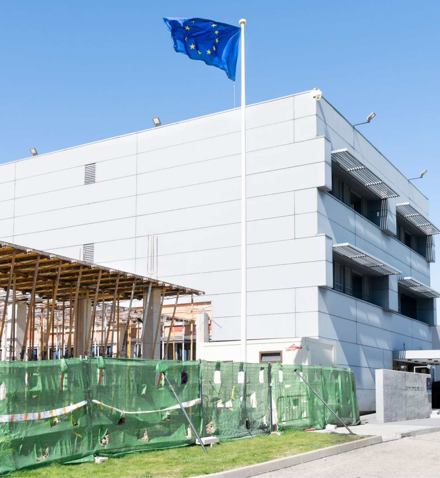
SatCen Headquarters in Torrejón de Ardoz, Madrid, March 2021 Construction site of the SatCen building extension, approved by the SatCen Board in 2018, started in December 2020 and scheduled to be completed in 2022.
